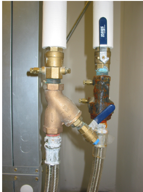
Figure 5.2. Heat pump hook up.
